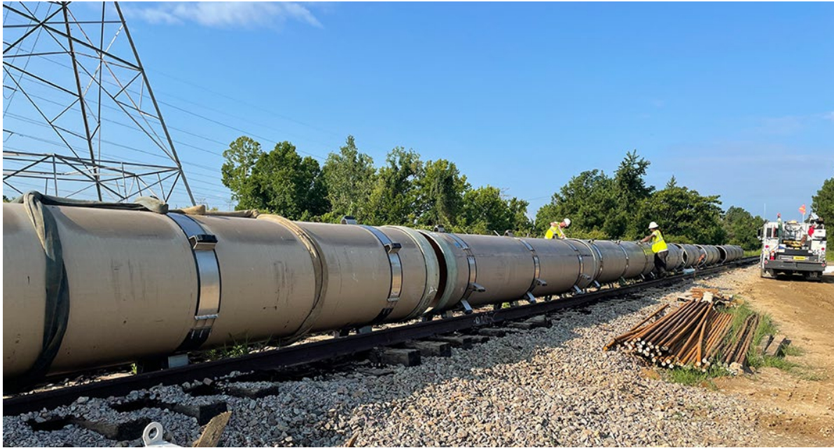
East Rocky Branch Sewer Improvements, Phase II Columbia, SC Completion Date: 2023 Size: 4,700 LF of 36-inch gravity; 2,500 LF of 42-inch gravity
