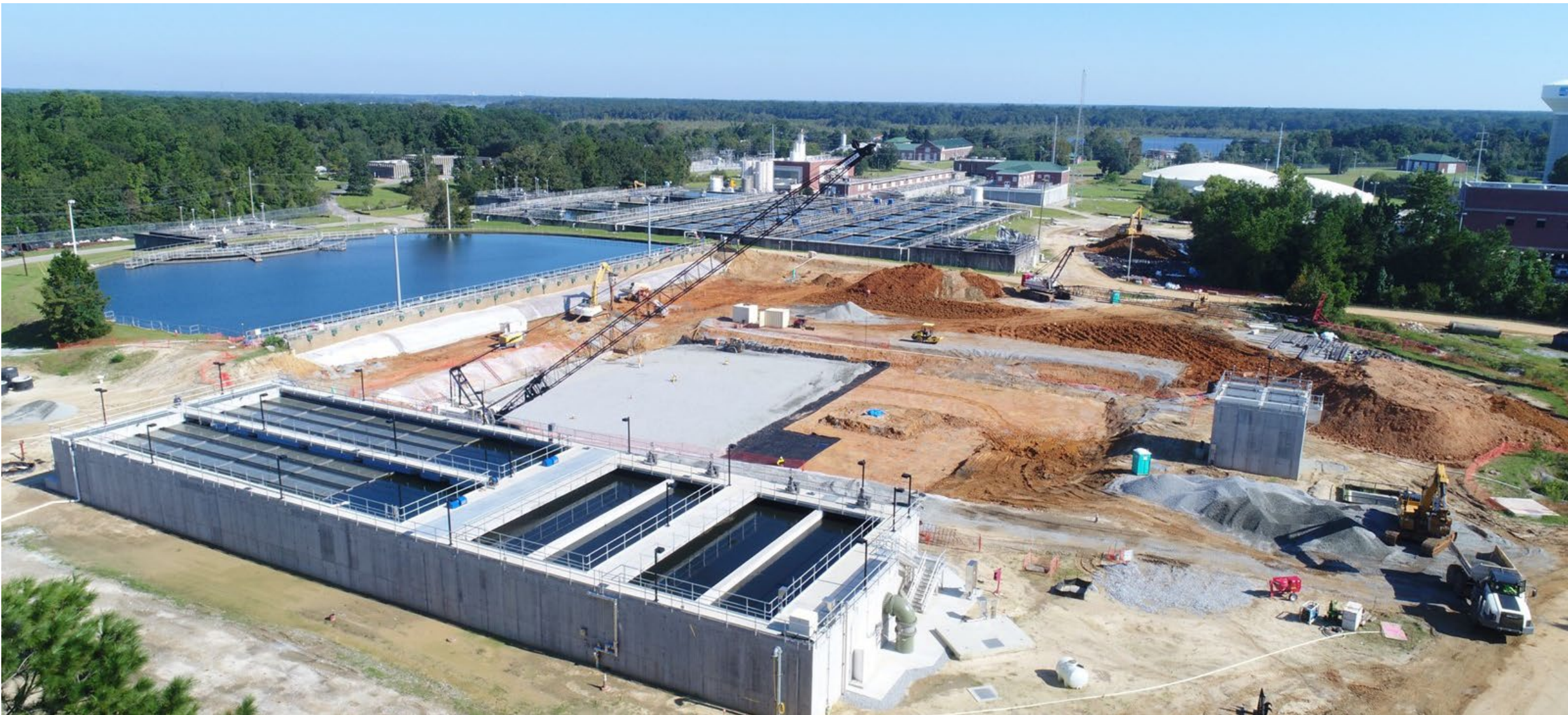
Charleston Water System Hanahan WTP Expansion, Charleston, SC Completion Date: 2030 est. (ongoing projects since 2014) Size: 127 MGD plant *Subconsultant to Black & Veatch for civil + survey services *Image courtesy of Black & Veatch
