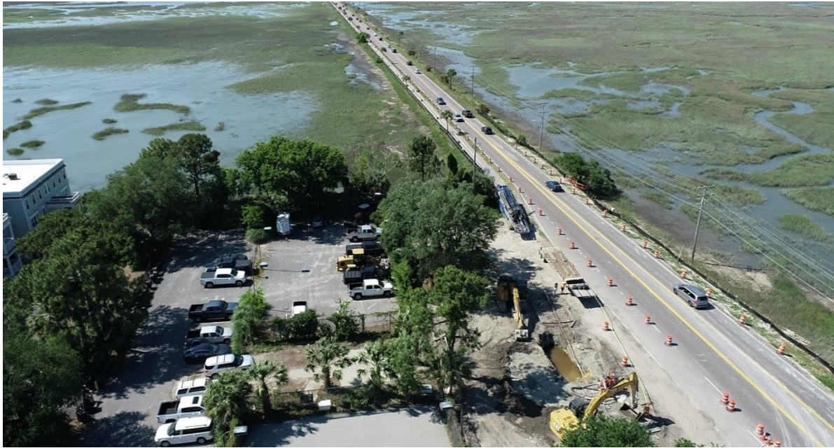
Ben Sawyer/Intracoastal Waterway Water Main Crossing Sullivan's Island, SC Completion Date: 2022 Size: 5,750 LF of 16" transmission water main
