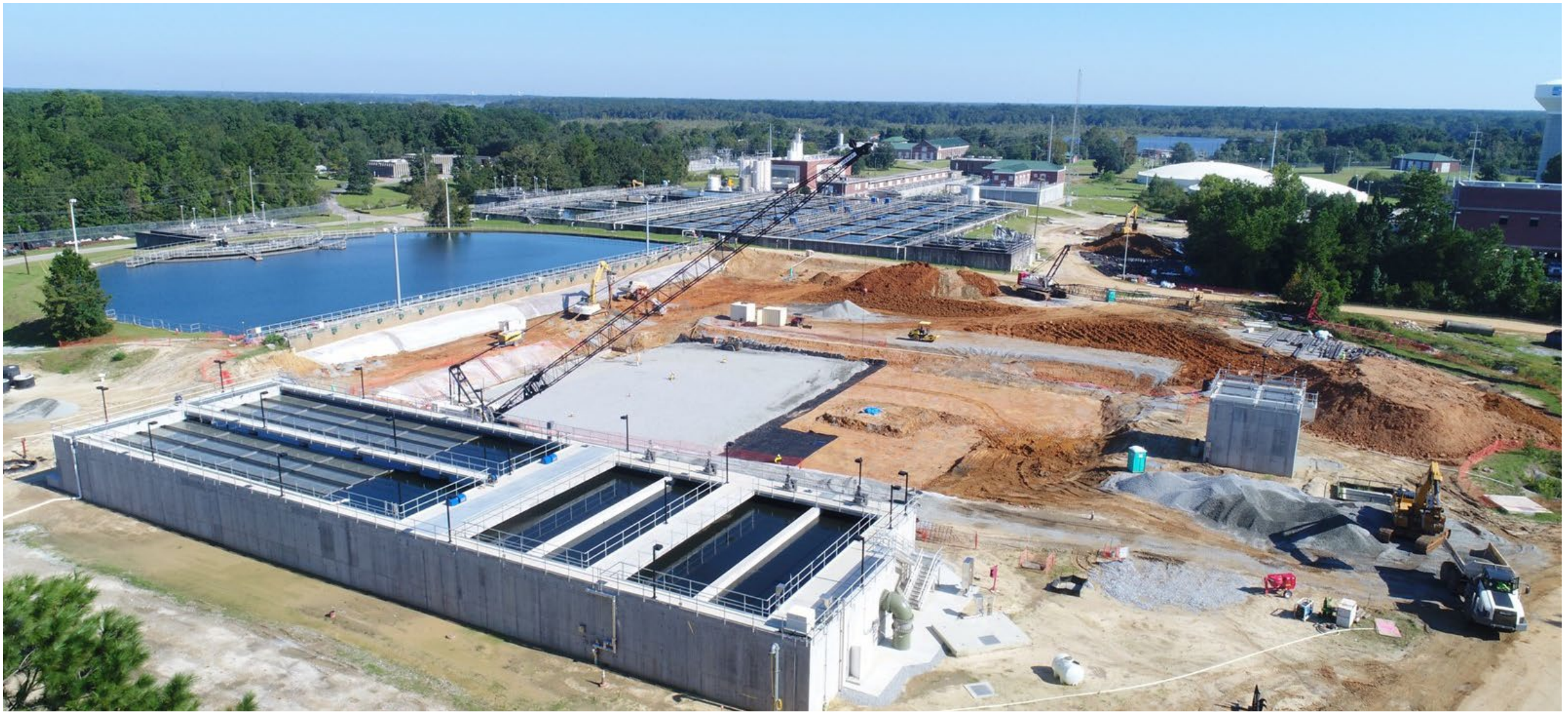
Hanahan WTP Expansion, Charleston, SC Completion Date: 2030 est. (ongoing projects since 2014) Size: 127 MGD plant *Subconsultant to Black & Veatch for civil + survey services *Image courtesy of Black & Veatch
